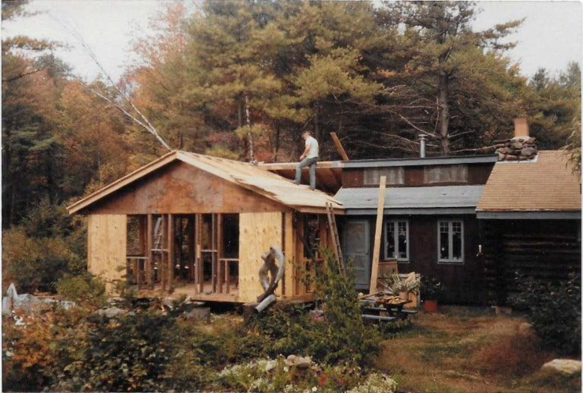
Fred Moller expanded a barebones cabin in Jaffrey into a large home with amenities like a library, root cellar and greenhouse. Courtesy photo
