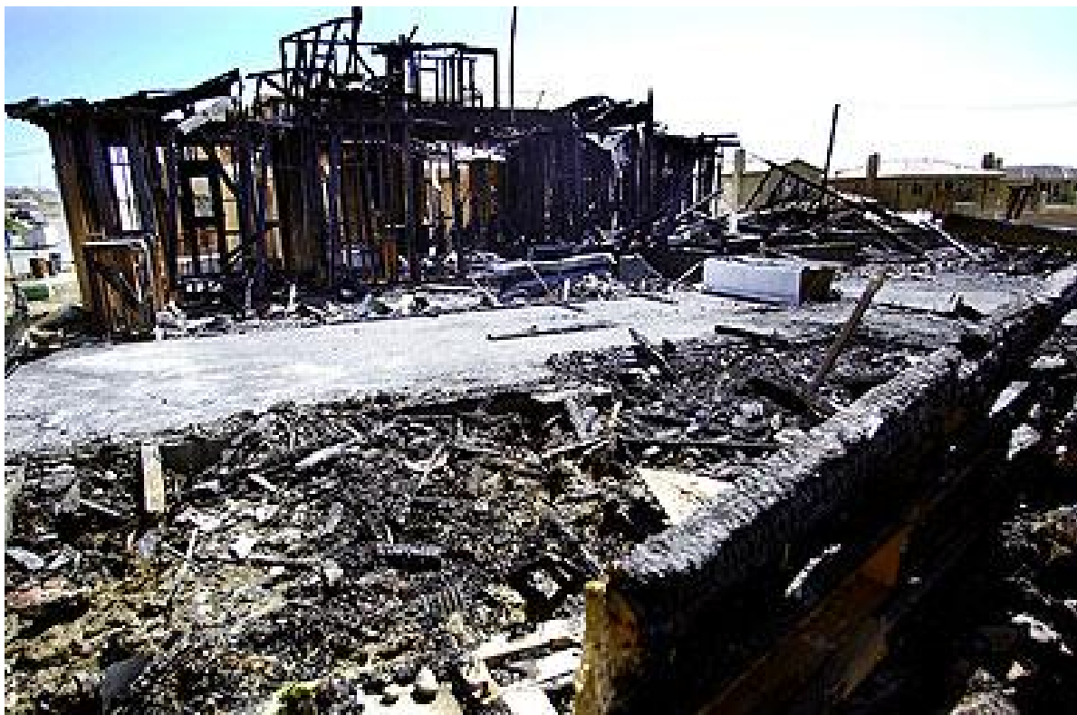
The remains of a new home construction site that was set on fire presumably by members of the Earth Liberation Front in San Diego, California.
